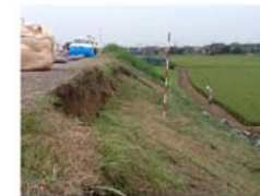
Photo 3. Site of sliding failure near KP8.4 on the right bank (MLIT, 2014)
