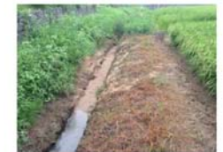
Photo 4. Sand boils near KP8.6 on the right bank (MLIT, 2007)
